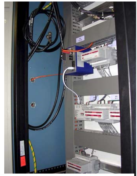
Industry-standard Ethernet fiber optic cable (orange) replaces proprietary coax
